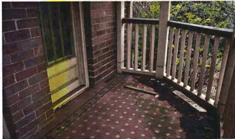
Figure 9 Detail view of the front verandah. The details appear to be contemporary to the construction of the house. Source Paul Davies Pty Ltd July 2009.
