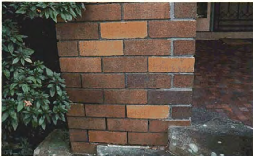
Figure 15 Detailed view of the front porch showing the stitch marks in darker mortar and bricks where the bay was removed to install the stone steps. Source Paul Davies Pty Ltd July 2009.
