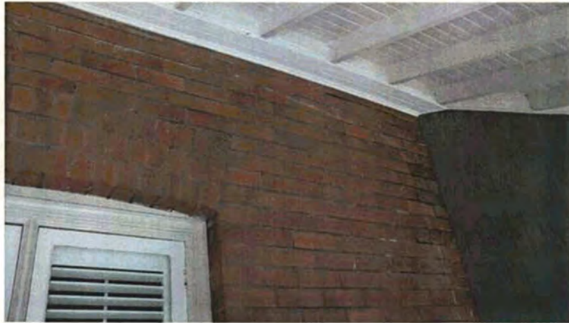
Figure 20 View within the front verandah of No 16 showing the silhouette of the original verandah post and beam. Source Paul Davies Pty Ltd July 2009.
