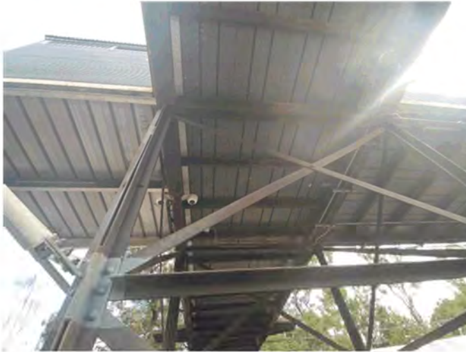
Figure 4-10 Steel substructure of footbridge and cantilevered kiosk. Note modern steel substructure of the footbridge deck (at left) (AECOM, 2021)
