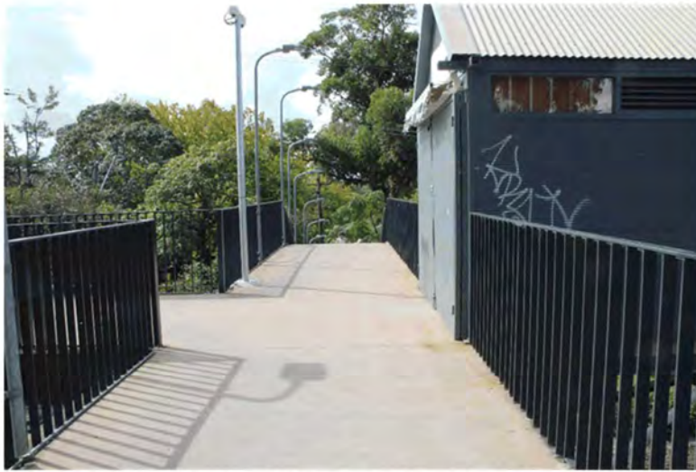
Figure 1-5 Deck of footbridge, looking east with cantilevered kiosk on the right (AECOM, 2021c)
