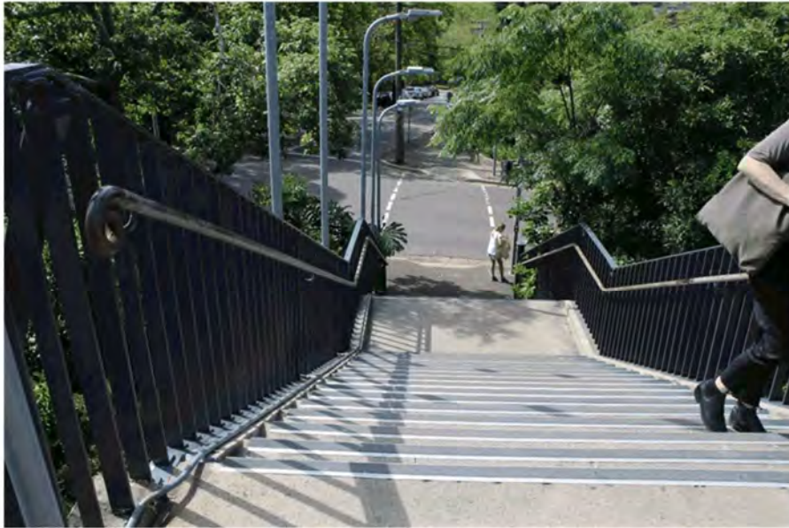
Figure 4-6 Stairs from footbridge to Werona Avenue. Note original tapered end of handrail (AECOM, 2021)
