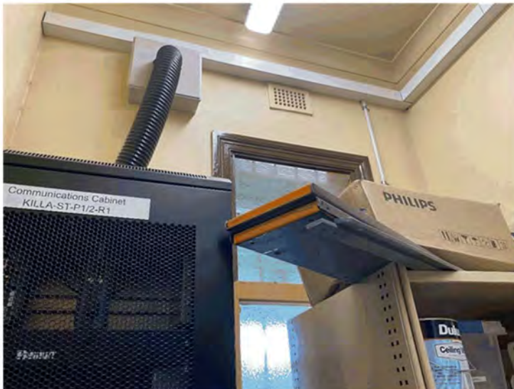
Figure 4-17 Western internal wall of communications/store room indicating original and updated features (AECOM, 2021)
