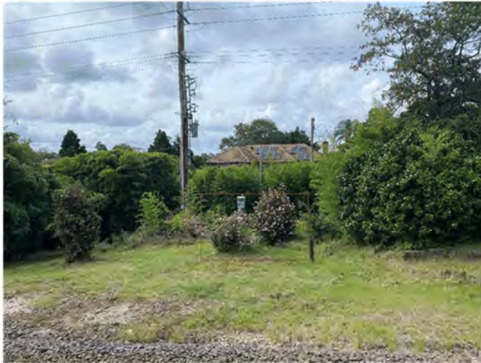
Figure 6-5 Location of transformer at the northern end of the garden; to be upgraded as part of the station power supply upgrade (AECOM, 2021)
