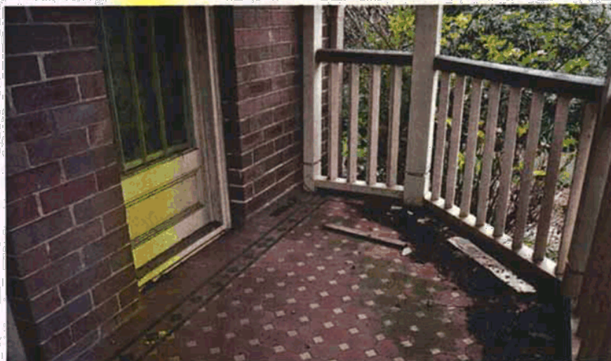
Figure 9 Detail view of the front verandah. The details appear to be contemporary to the construction of the house. Source Paul Davies Pty Ltd July 2009.
