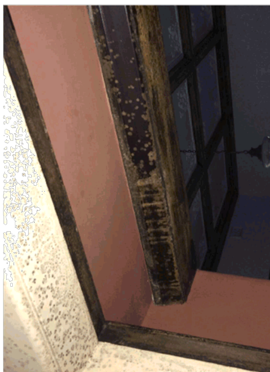
Details of steam and mould damaged fabric
