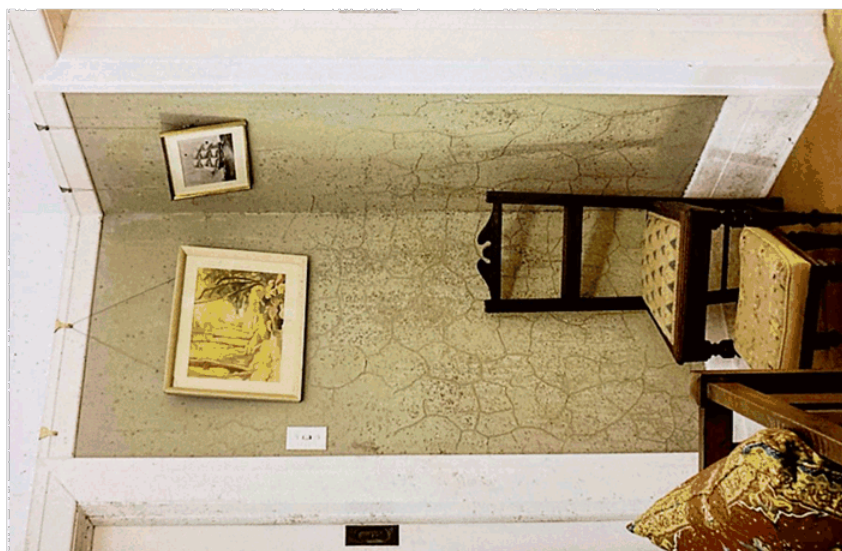
Morning room: Damage and restored
