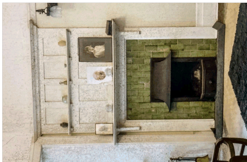
Living room: Damage and restored
