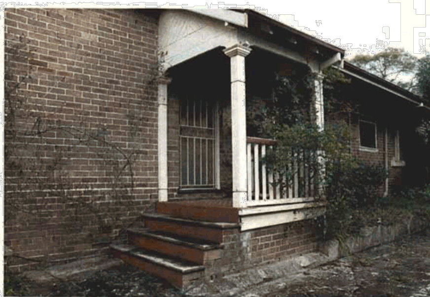
Figure 10 Figure 11 View of the interior of the side porch. The details appear to be contemporary to the construction of the house except for the poorly fitted treads and risers. Source Paul Davies Pty Ltd July 2009.
