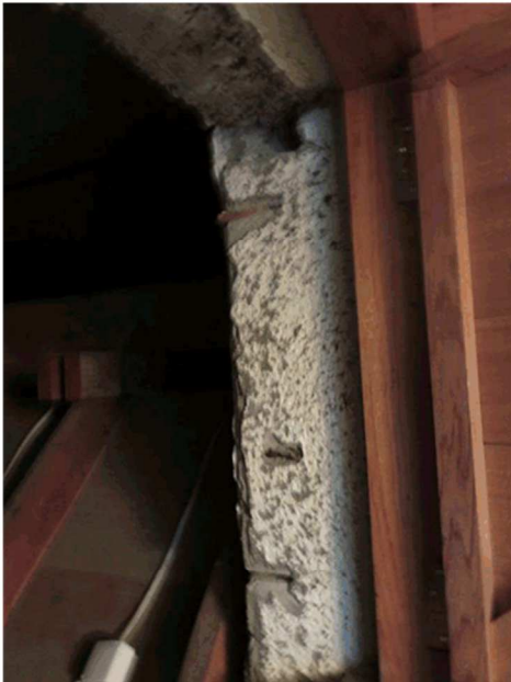
Figure 3.42 When opened the access door allows for views of the building's original external stucco finish and the space above the ceiling of the chapel. (Source: GML 2017)
