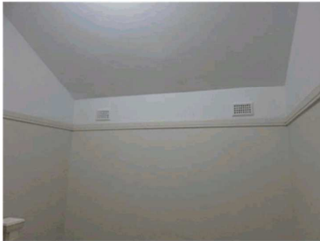
Figure 3.34 The upper part of the eastern wall of the upper landing, above the stair. The air grilles suggest this was originally an external wall. (Source: GML 2017)
