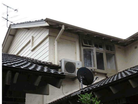
Figure 3.17 The original timber window that exists in the upper part of the east elevation of the main part of the building. The boarded gable of the south elevation can be seen on the left. (Source: GML 2017)
