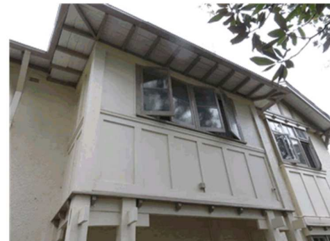
Figure 3.11 The verandah above the entry porch. The windows are a later addition. (Source: GML 2017)
