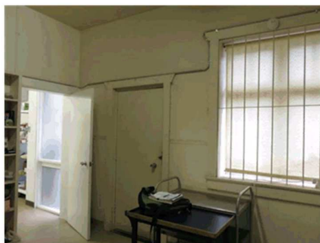
Figure 3.33 The southeastern corner of the shop store. The door on the right leads outside. (Source: GML 2017)
