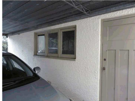
Figure 3.15 The south elevation of the garage, with door and window that are likely to have been salvaged from elsewhere on the site. (Source: GML 2017)
