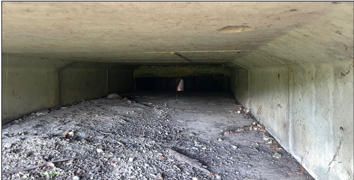
Figure 6. Box culvert identified within the eastern extent of the Subject Site which may provide potential roosting habitat for Microbats.
