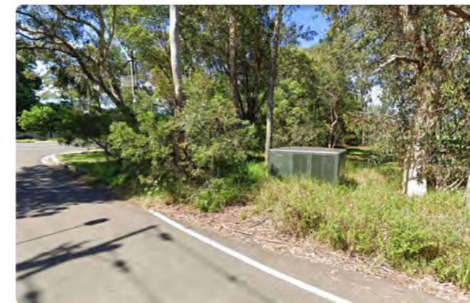
Electricity substation located on Palm Street
