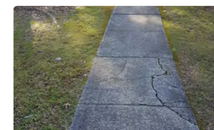
Existing path deterioration
