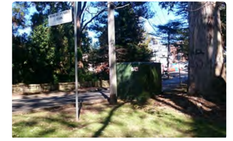
Electricity substation located on Alma Street
