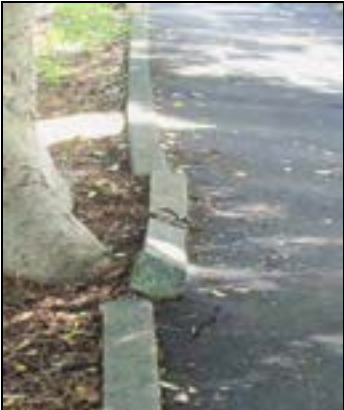
Root damage to kerb and edges
