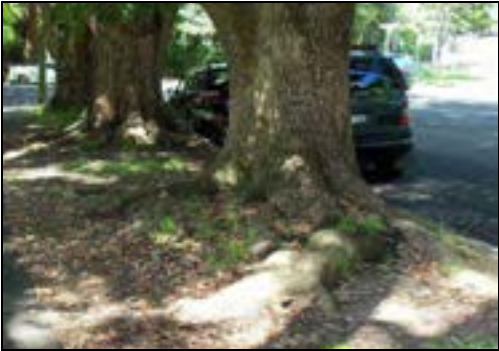
Surface root damage
