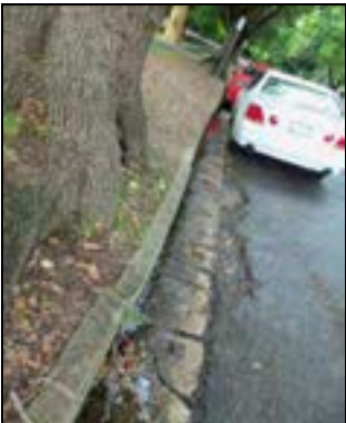
Root damage to gutters and drainage
